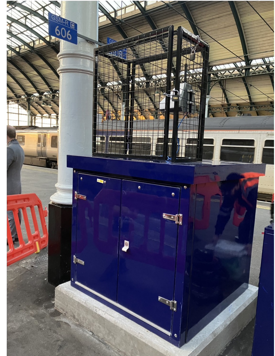
Photo: Air quality reference monitor being installed at Hull Paragon Station.
