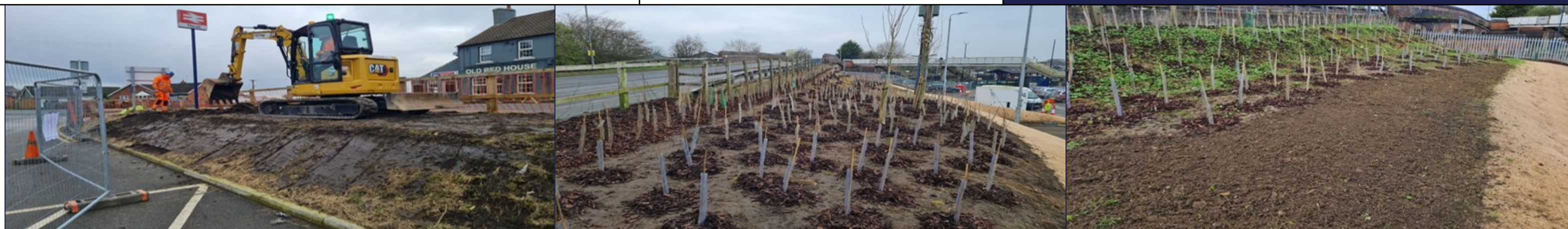
Photos: Thirsk station embankment reprofiling, new scrub and hedgerow planting on the embankment and area prepared for wildflower seed mix.
